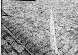
Section B - Deficiency #3 Deteriorated valley tin
