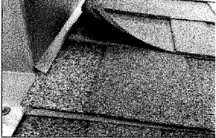
Section B - Deficiency #5 Poorly installed flashing
